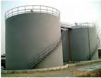
12 Meters Bitumen Tank
