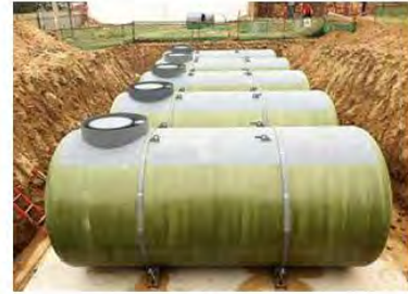
2 Meters Underground Tank
